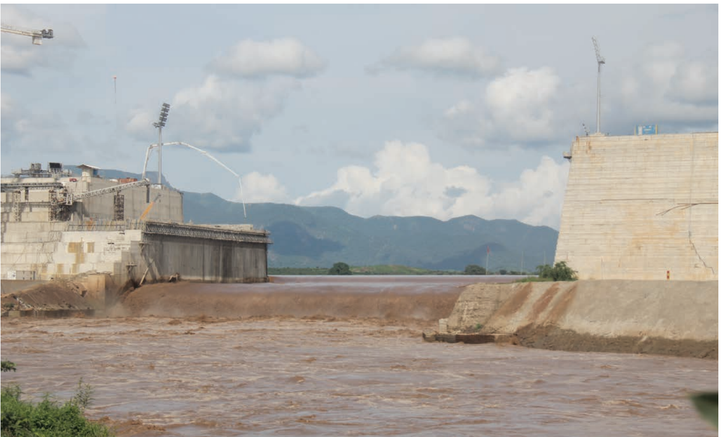
> OPEN SPILLWAY OF THE GERD CONSTRUCTION PROJECT. The sill level will be incrementally raised throughout the filling process and releases can be made through the turbines, via the bottom outlets and over this spillway. © Kevin Wheeler
