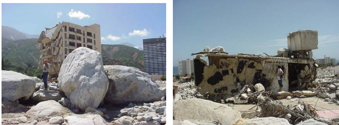
Figure 3. Damages by debris flows to two buildings on the alluvial fan of San Julian River.
