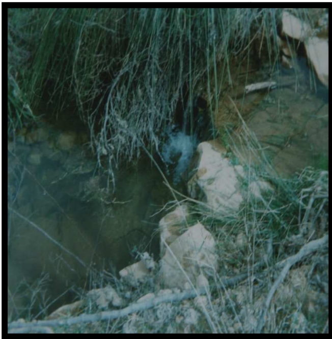
Photo 3. Water leakages the level of left bank Beside piezometer SB13. Dam Ouizert ( q )
