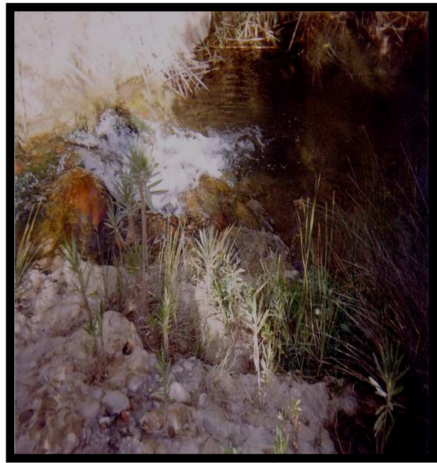
Photo 4. Place of meeting held on the three water leakages on the level left bank. Dam ouizert (S)
