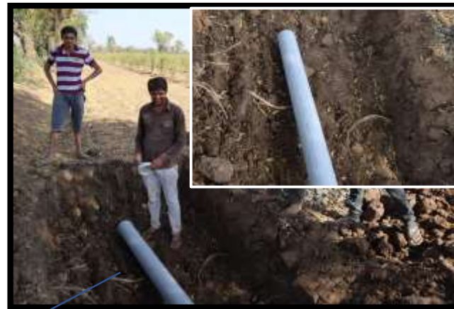
Slitted Pipe to be Placed under a pit that is covered by ballast and sand at the sink point to divert the rainwater flowing out of the fields.
