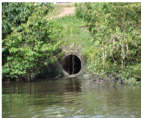
Figure 12. Wastewater discharge into Sanhauá river indirectly through pluvial drainage system
