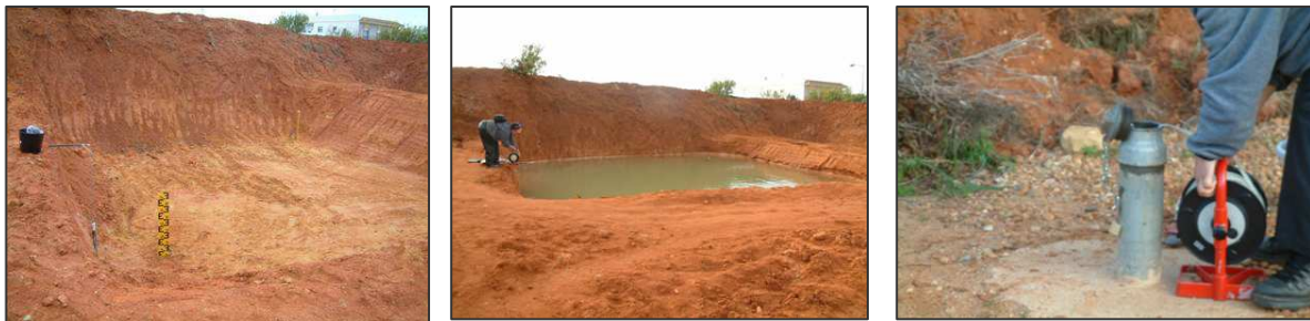
Figure 10 – Infiltration basin in the second layer and monitoring equipment used for the infiltration test
