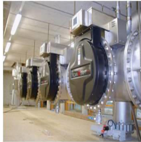
Andijk drinking water treatment plant in Netherlands
