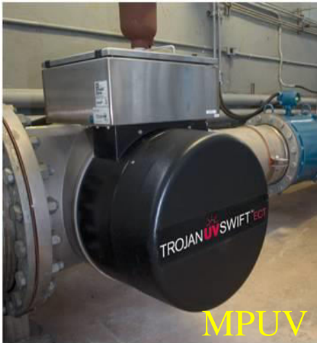
Cornwall drinking water treatment plant in Canada
