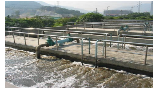
Municipal sewage treatment plant
