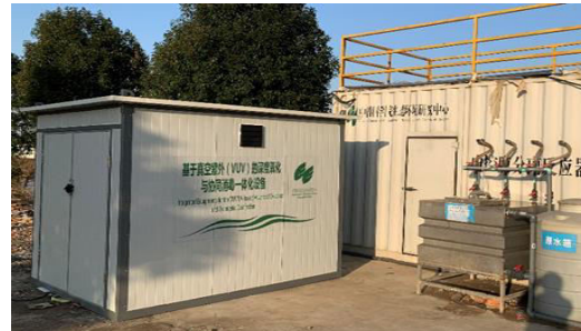
Rural drinking water treatment facility
