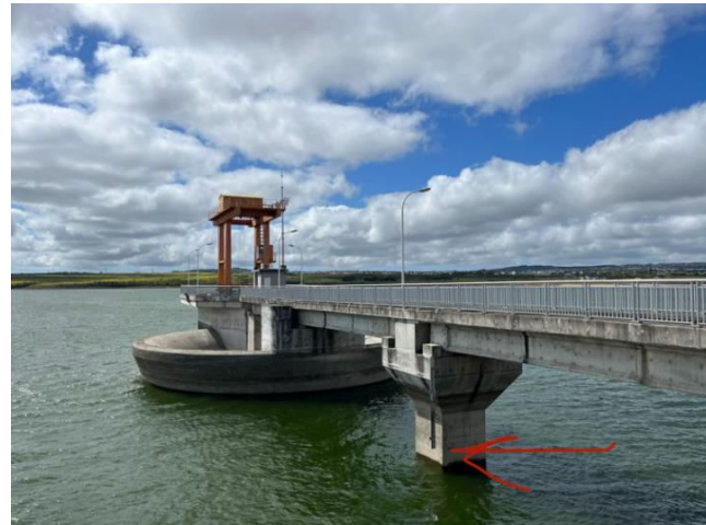
Water meter is not touching reservoir surface in Mauritius (credits: Y. Vystavna)
