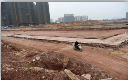
soil erosion and sediment accumulation
