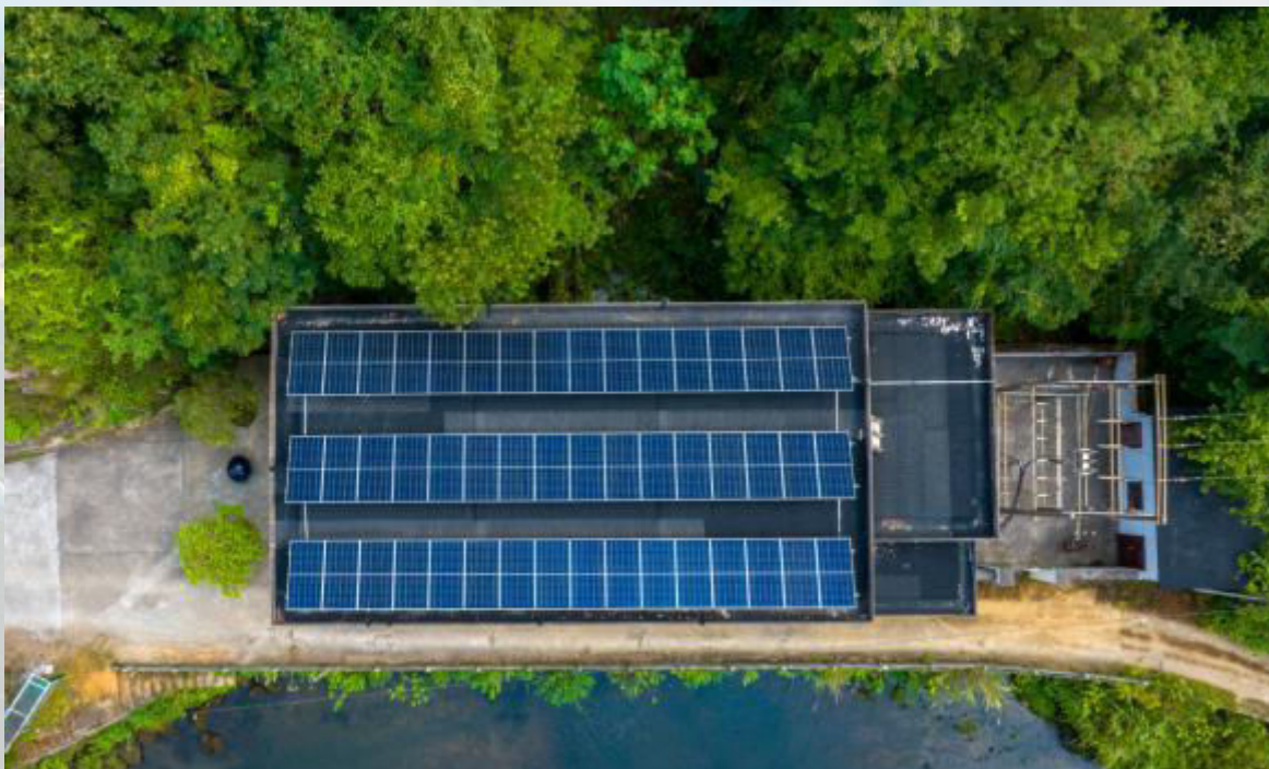
藏潭桥水电站屋顶光伏现场图 Roof photovoltaic scene of Zangtanqiao Hydropower Station
