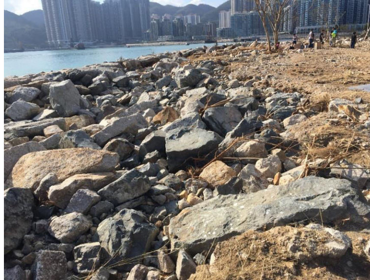
Damage of waterfront promenade by wave overtopping during Mangkhut
