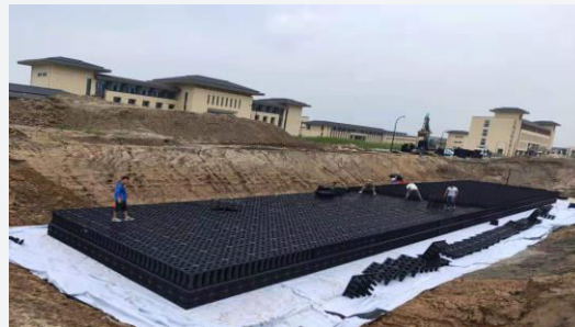
Rainwater collection pool
