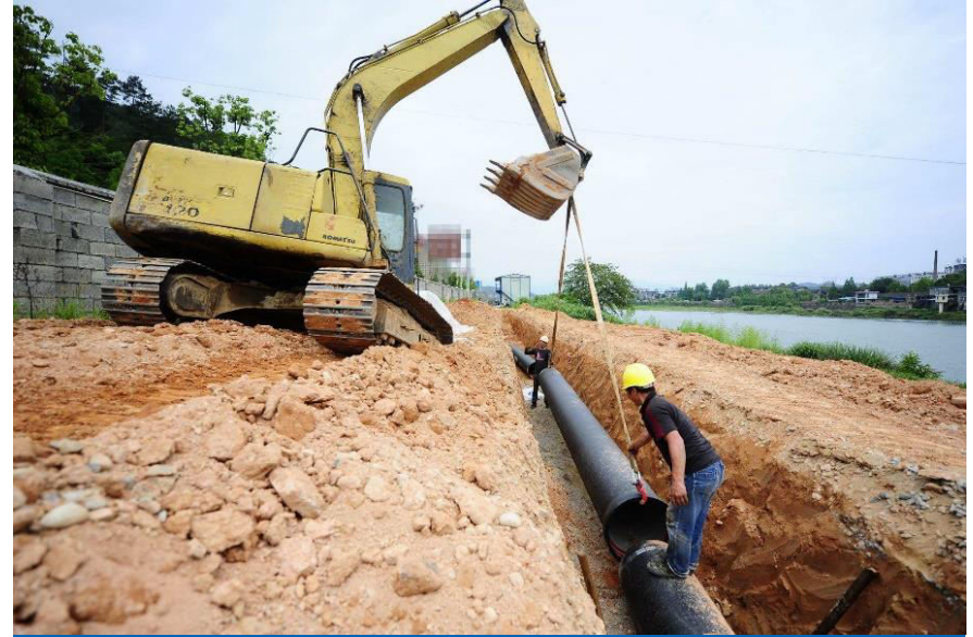
Drainage system needs improving
