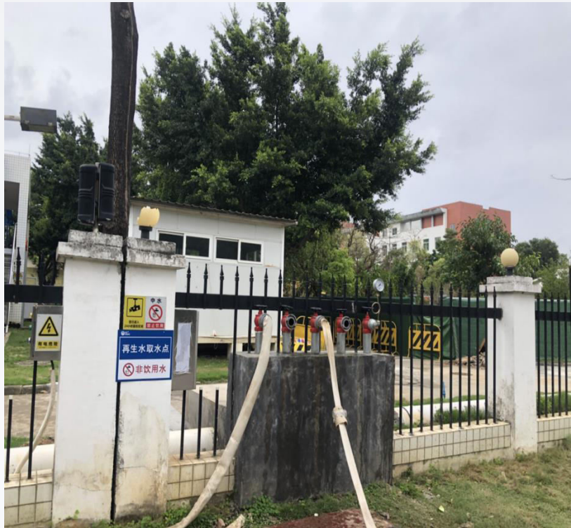
Municipal water intake point (市政取水点)
