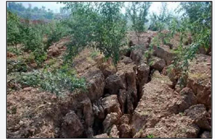
Ground crack (Longyao)
