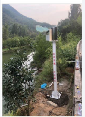
Automatic Monitoring (56067 Rain-gauge and 22562 stage gauge)
