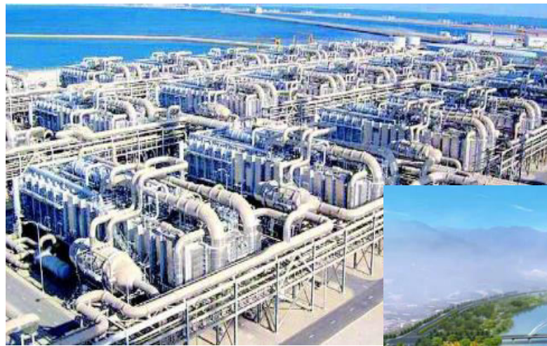
Sea water desalination
