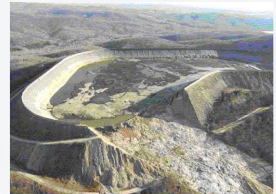
Upper Taum Sauk dam breached (2005.12.14)
