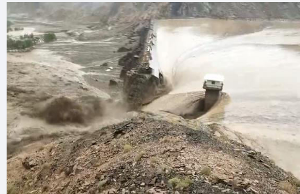
Sheyuegou core dam breached (2018.7.31)
