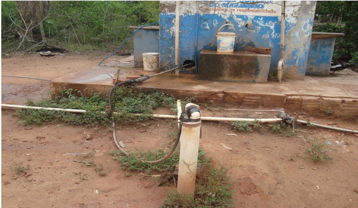
Figure 9 – A leak at the discharge outlet of the well, fixed with strips of rubber. Note as well, that at this well there is both an area to fill up buckets for the population to take water to their homes and at the same time sinks to wash dirty laundry.
