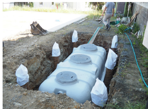
Fig.23 5.6 tons rainwater tank
