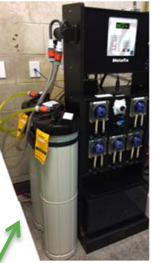
Rinsing water quality control unit system
