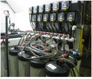
Two industrial scale installations
