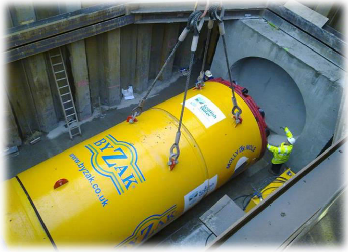
Large diameter tunnels
