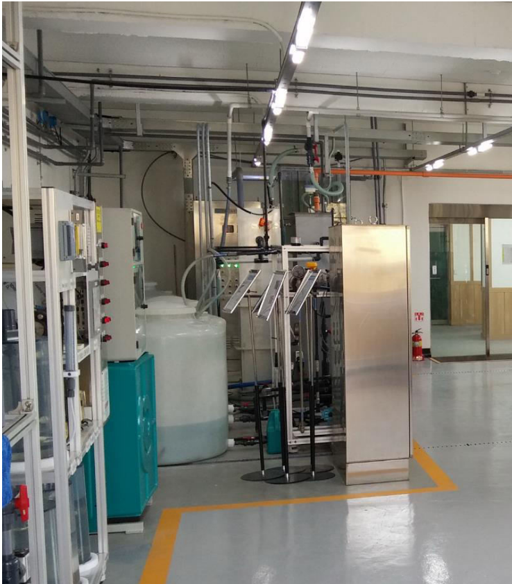
Smart Water Grid Pilot Plant in Bupyeong WT
